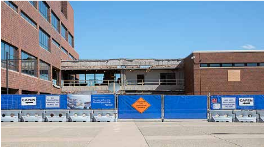
A view of the One World Café construction site from Flint Loop showing the exposed south side of Norton Hall (Meredith Forrest Kulwicki)
